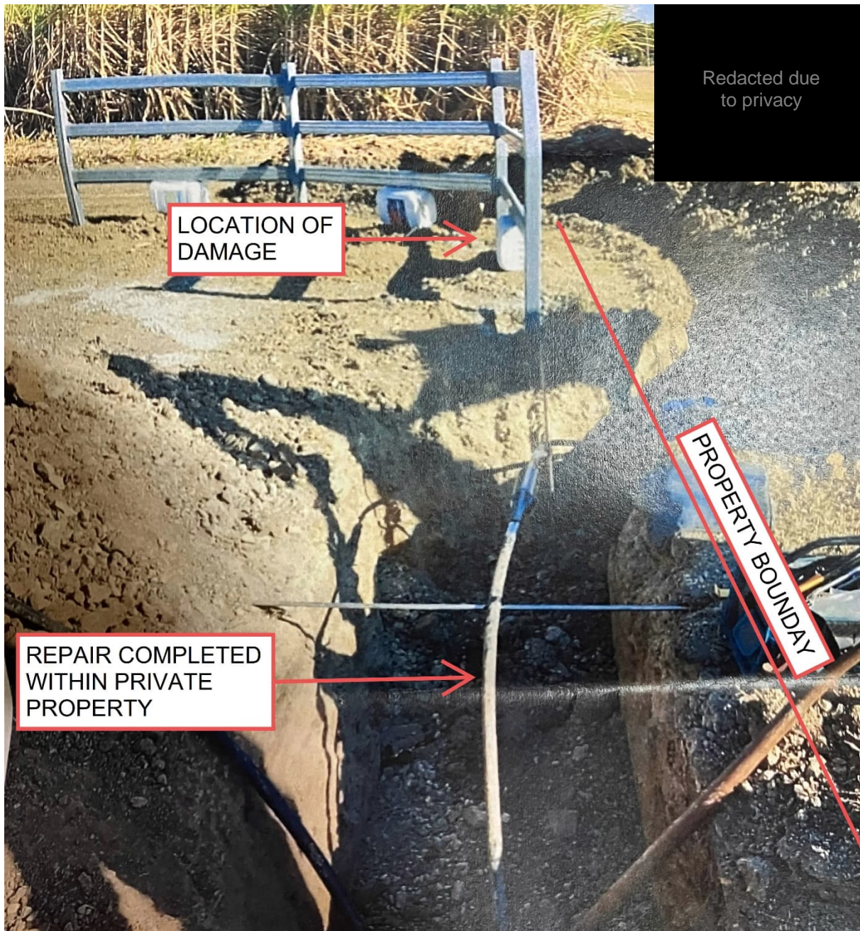
Figure 14 Telecommunication Service Severance and Repair
