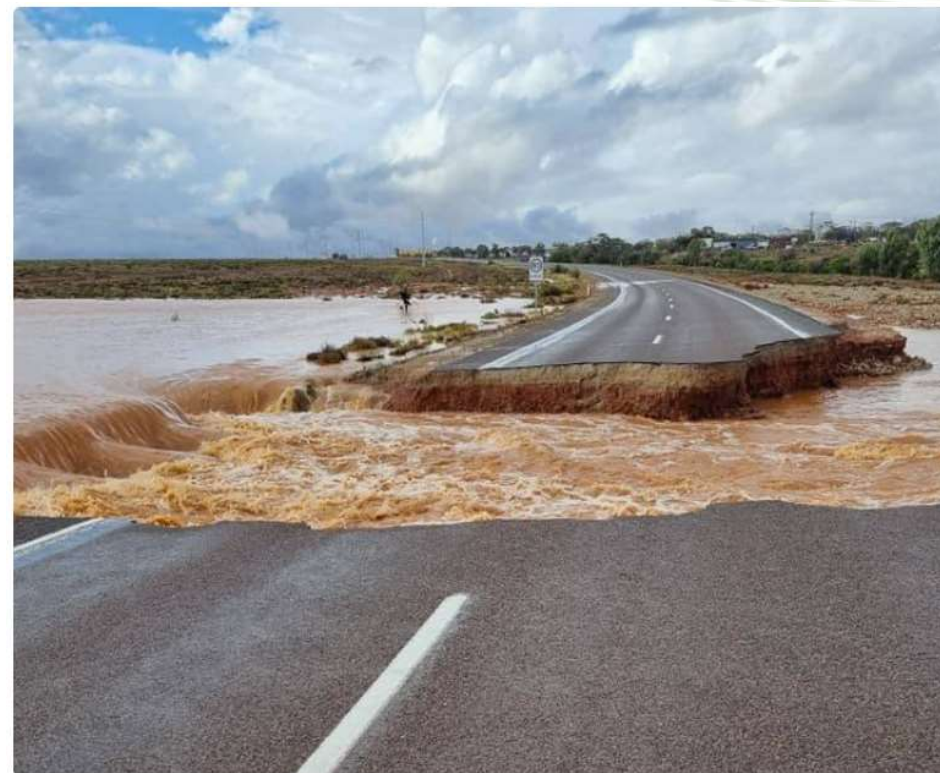
Figure 5 - Sturt Highway Damage - Picture: Spuds Roadhouse
